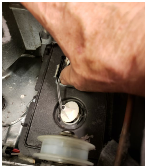
Figure 17, Partially-seated float switch for the malfunctioning heat pump dryer at Site 1.
