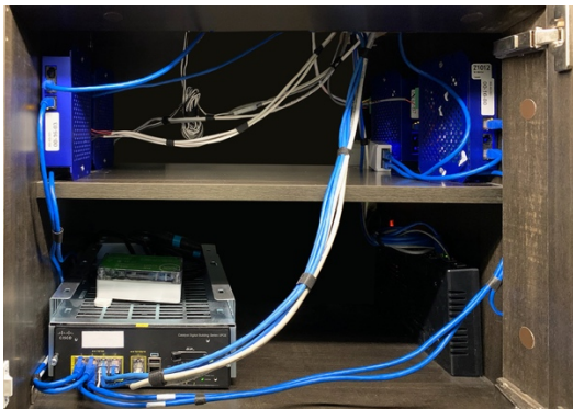
Cisco CDB UPoE network switch powering the PoE devices in a guest room at The Sinclair.
