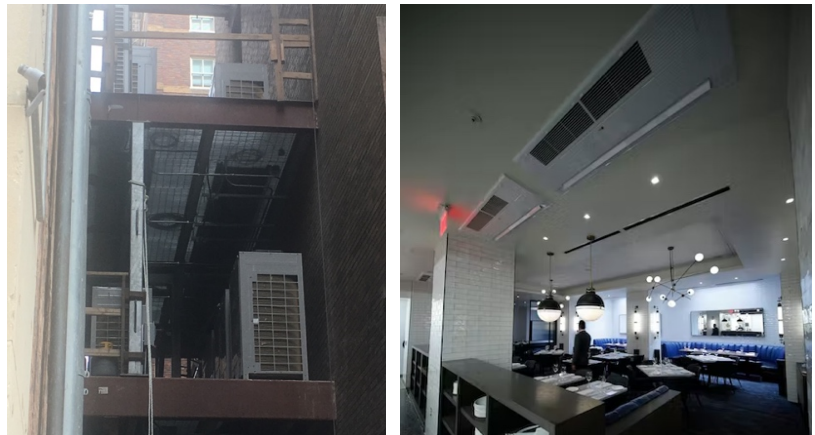
Condensing units of the VRF System and VRF Cassettes in the hotel basement restaurant.
