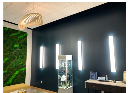
PoE lights in the SPPA Reception area.
