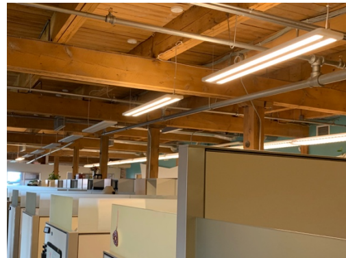
PoE lights in CEE's Admin office area.
