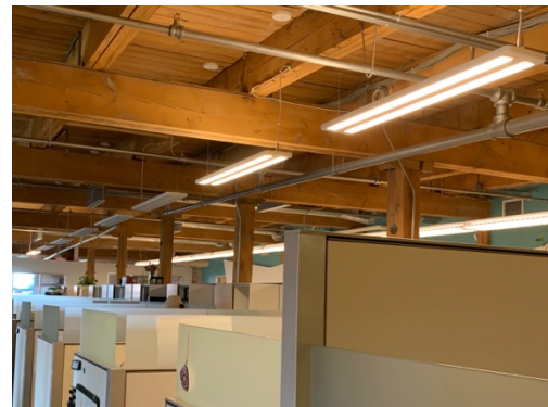
PoE lights in CEE's Admin office area.
