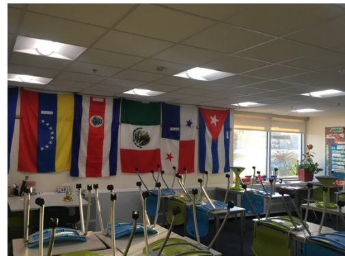
Edina, MN's South View Middle School classroom uses PoE lighting.
