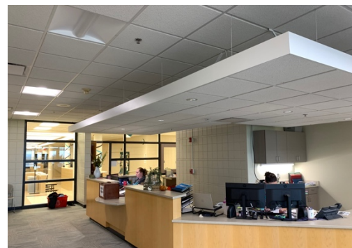
PoE lights in the Admin Office of the ACGC Junior/Senior High School.
