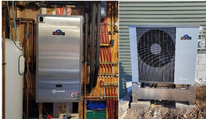
Figure 4: The Enertech Advantage AV060 IDU (left) and ODU (right) as installed at site 3
