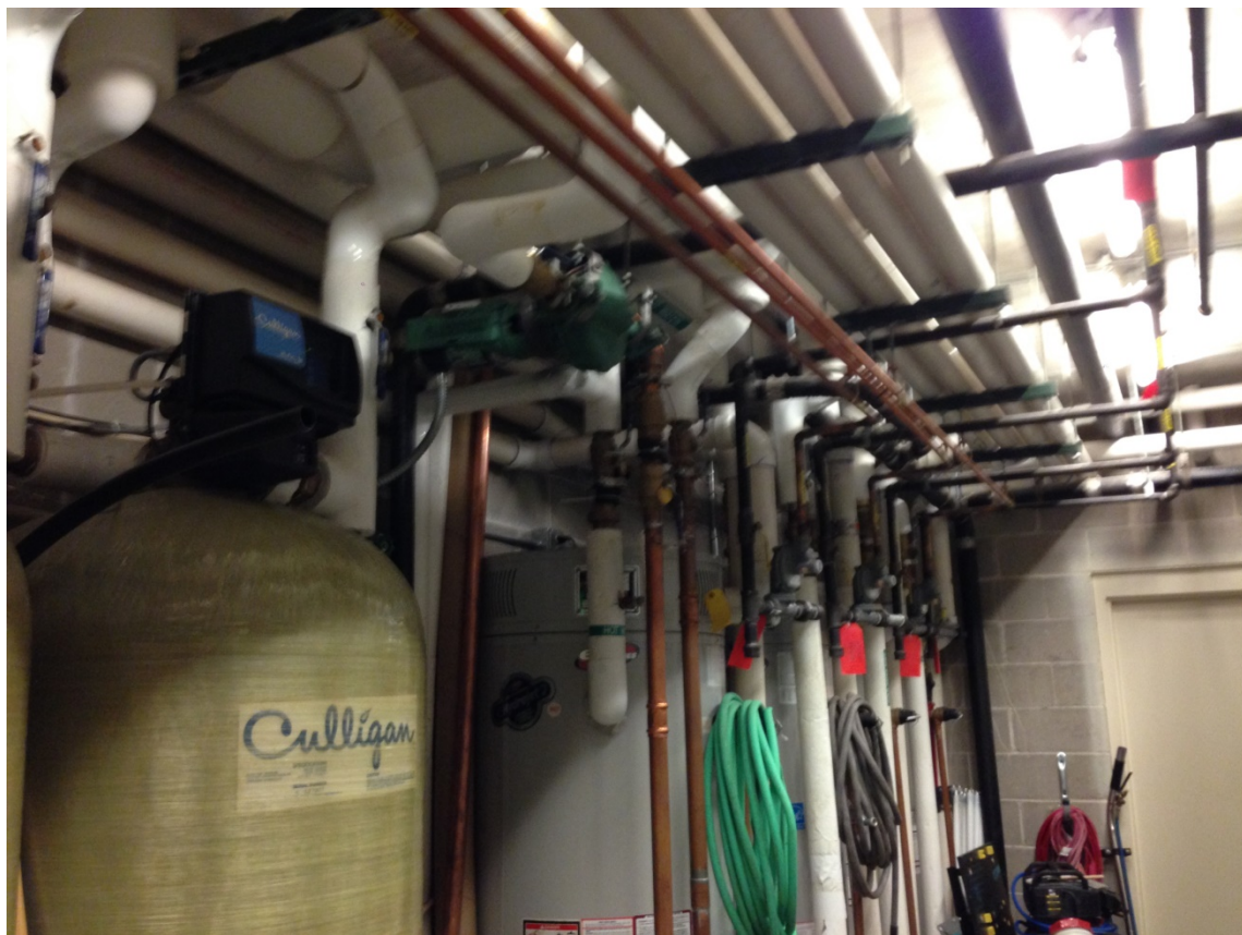
Figure 11. Central DHW area of the mechanical room at Hosp_2
