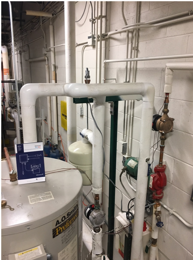
Figure 38. Water heater and recirculation pump at Com_3
