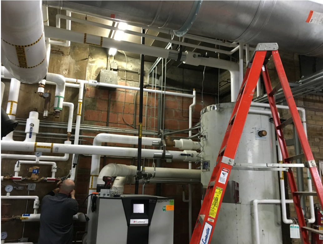
Figure 22. Water storage tank and boiler at Com_Ed_1
