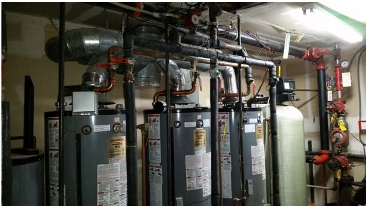
Figure 16. Water heating area of the mechanical room at Hosp_3
