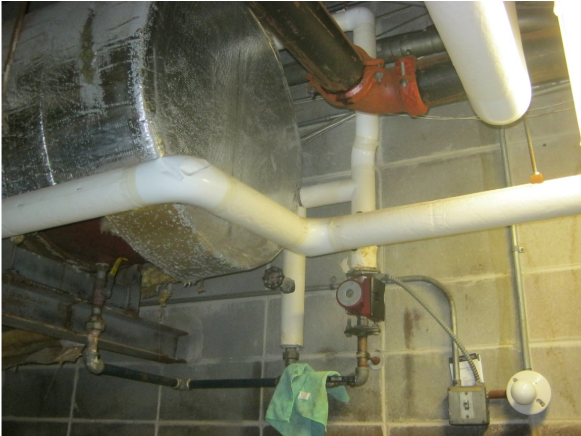
Figure 26. Indirect storage tank and recirculation look at Com_Ed_02
