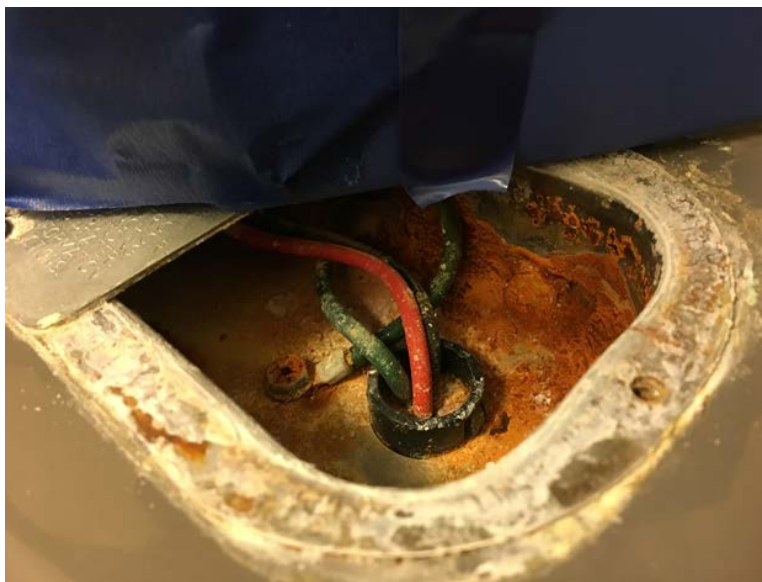
Figure 49. Site E01 - M&V Sensor Leaks
