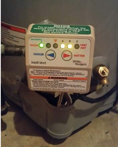
Figure 51. Site G14 - Failed Gas Valve
