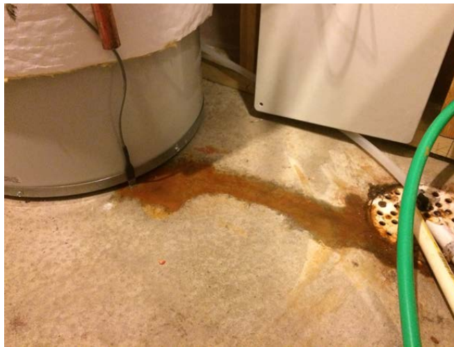
Figure 50. Site E05 - Water Heater Leak
