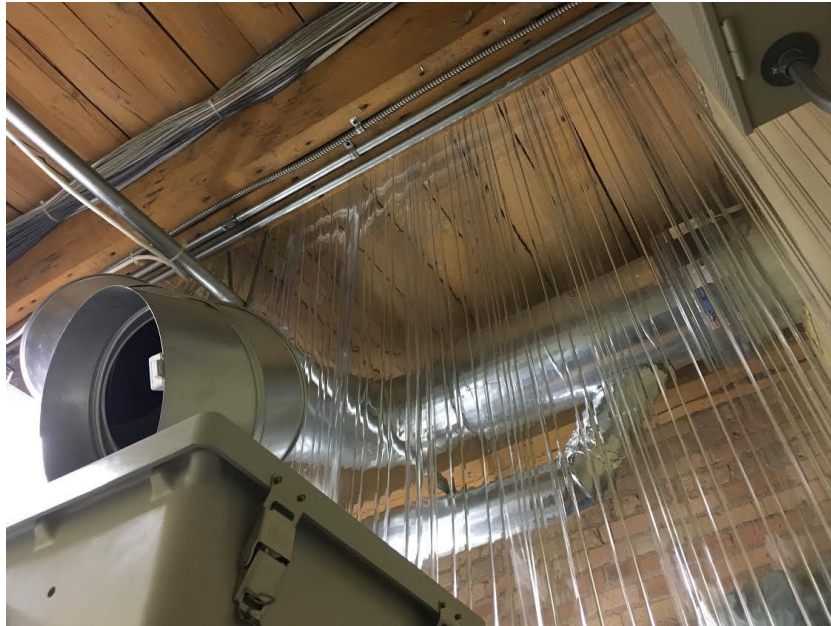
Figure 68. Drapes at Site 6 Enclosing the Exhaust Fan in the Hot Aisle
