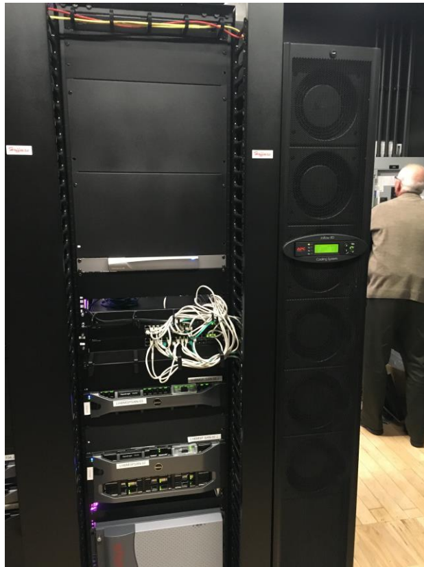
Figure 29. In Row CRAC at Site 2
