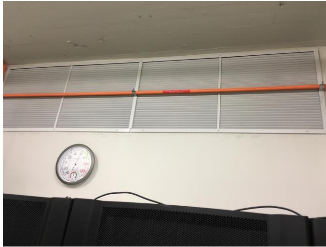
Figure 28. CRAC Return Grilles at Site 1
