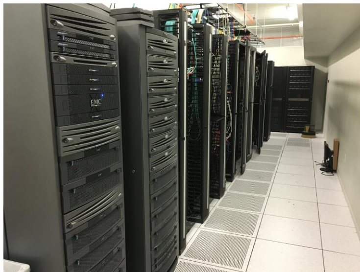
Figure 55. Server Racks at Site 1
