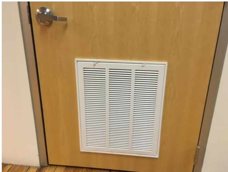
Figure 71. Supply Air Inlet to Site 6 SEDC
