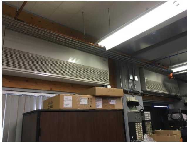
Figure 34. Ductless Splits at Site 8
