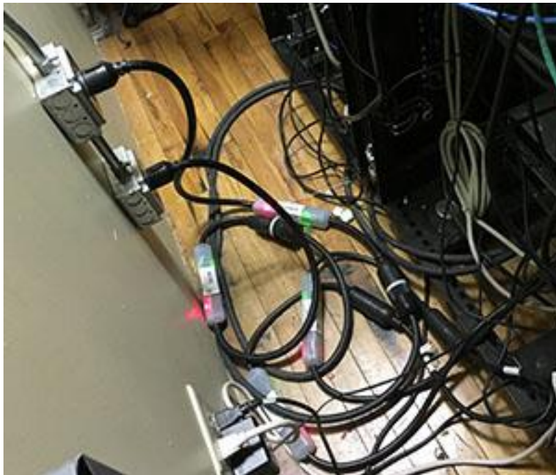
Figure 13. Site-Installed Packet Power Cables
