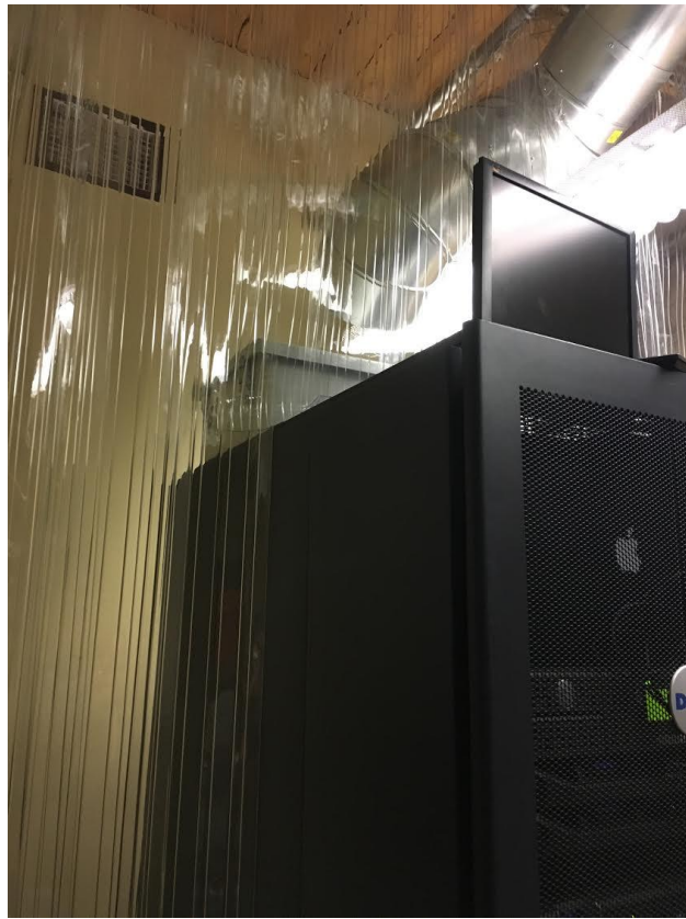
Figure 67. Plastic Drapes Partitioning a Hot Aisle in the Site 6 SEDC
