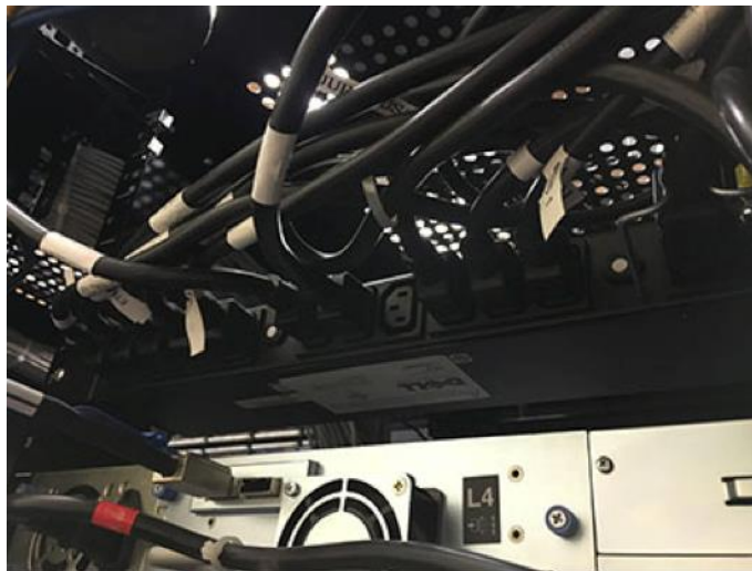
Figure 5. Power Distribution Unit (PDU)
