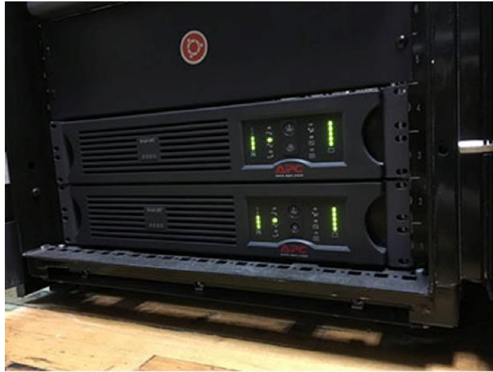
Figure 4. Two Rack-Mounted UPSs
