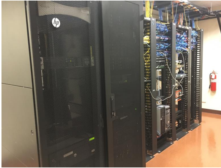
Figure 24. Server Room at Site 5
