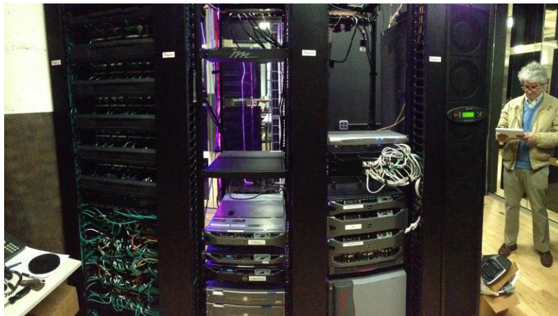
Figure 58. Server Racks and In-Row CRAC at Site 2
