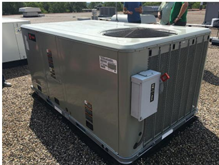
Figure 8. Roof Top Unit (RTU)
