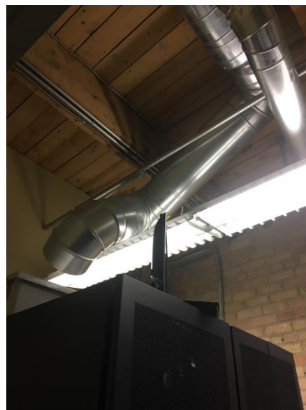
Figure 35. Ducting to Exhaust Fan at Site 6
