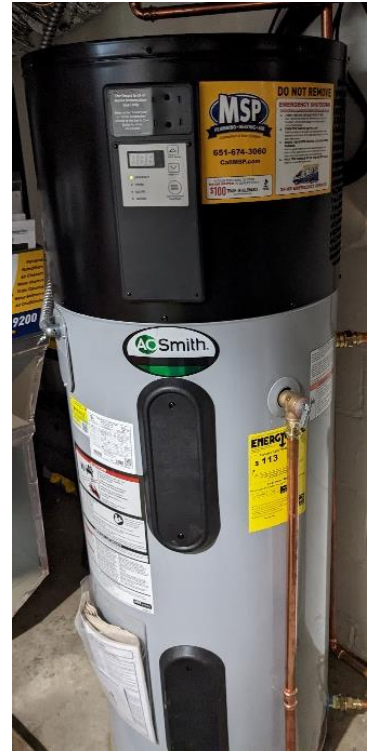
Heat pump water heater
