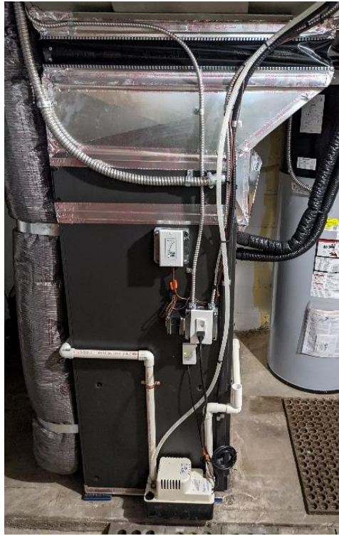
Heating system air handler
