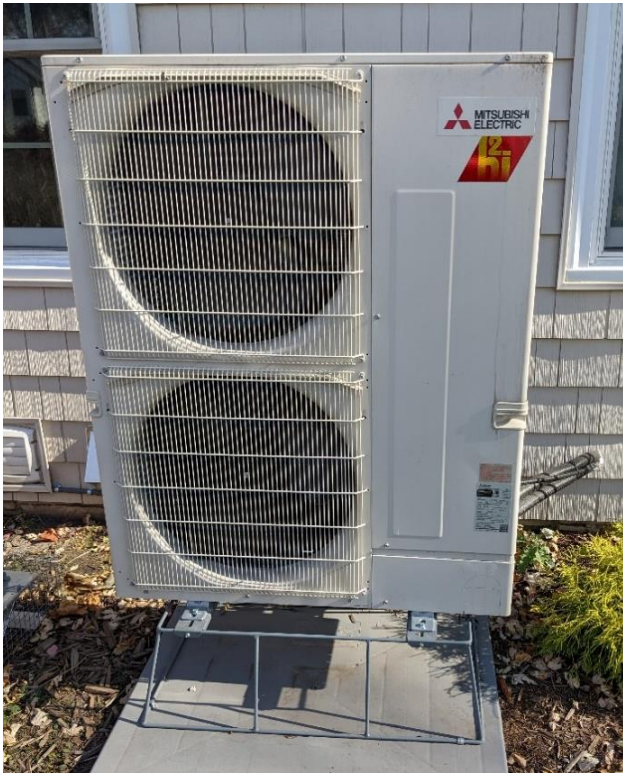
Air source heat pump outdoor unit
