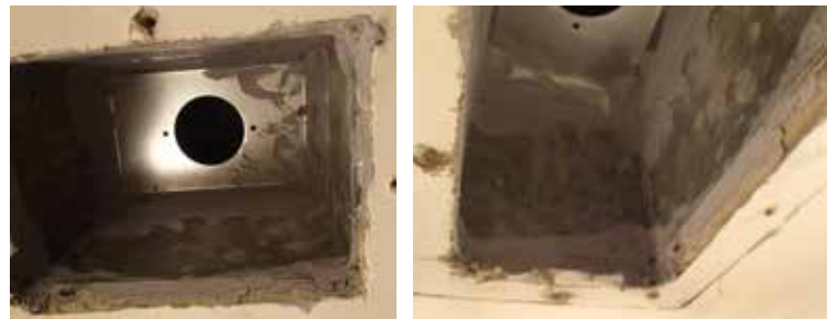
Figure 11: Left image - new fixed inlet orifices installed. Right image - register grilles were removed, the old balancing louvers were detached and discarded, the new balancing orifices were installed, and mastic sealant was applied to any leakage around the orifice and at the ceiling connection.
