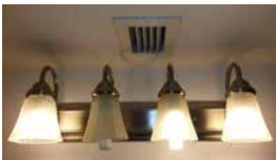
Bath exhaust inlets. Each bath had a 4"x6" inlet with a balancing damper behind the grille to control exhaust flow. The building had a mix of one and two bathroom apartments.
