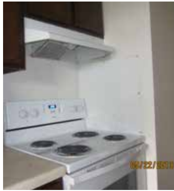
Figure 4: Kitchen exhaust inlets. The exhaust hood over the stove is connected to a continuous PRV fan. It can also be switched on at the exhaust hood to boost already high flows to double or triple their rates.
