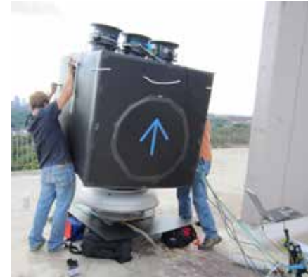
Figure 5: A collapsible capture cube fitted with 3 Duct Blaster fans was set over exhaust fans on the roof, measuring flow when the pressure in the cube matched the shaft pressure. A comparison of the total flow of all inlets on a shaft to the outlet flow for that shaft gave an indication of the amount of duct system leakage.
