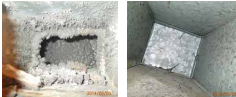
Figure 12: Branch ducts at bath inlets before and after cleaning. Branch duct inlets were cleaned before the new balancing orifices were installed.
