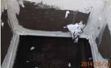
Mastic applied to curb below PRV fan to provide an airtight connection between ventilation shaft and fan.
