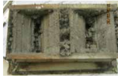
Figure 10: Clogged balance louvers.
