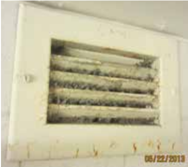
Partially clogged bath inlet fan.
