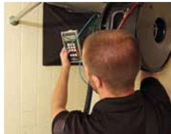
Figure 6: Bath inlet measurement. The FlowBlaster adapter for the DuctBlaster fan, measures inlet flow accurately on central exhaust systems by utilizing the calibrated DuctBlaster to compensate for pressure drop from the capture hood.
