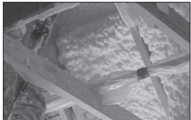
Figure 16. Applied spray foam at the underside of the roof sheathing. Demilec (USA) LLC® spray foam. Photo courtesy NEXUS EnergyHomes, Inc.
