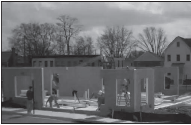
Figure 15. Construction phase at North Pointe, showing Murus® Structural Insulated Panels. Photo courtesy NEXUS EnergyHomes, Inc.
